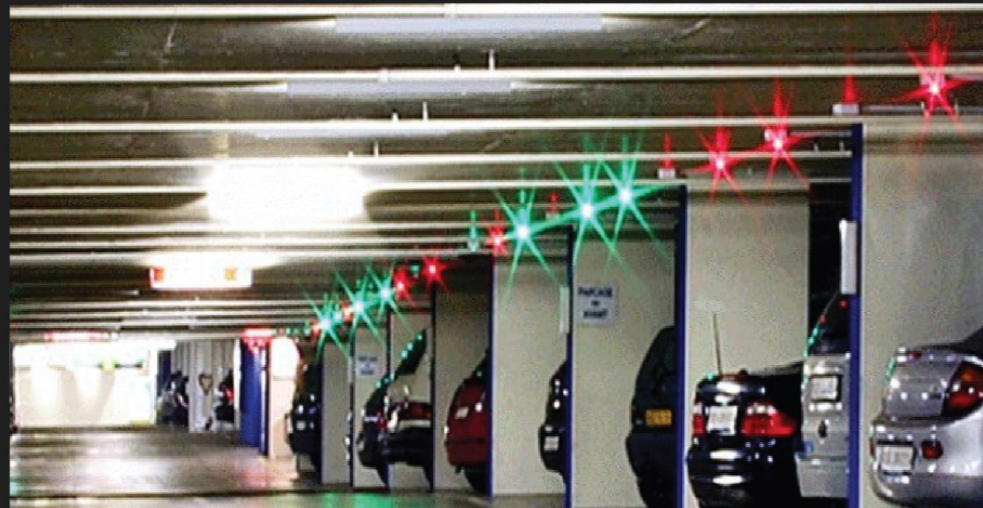
DEDICATED CAR PARKING MANAGEMENT SYSTEM FOR RETAILERS
